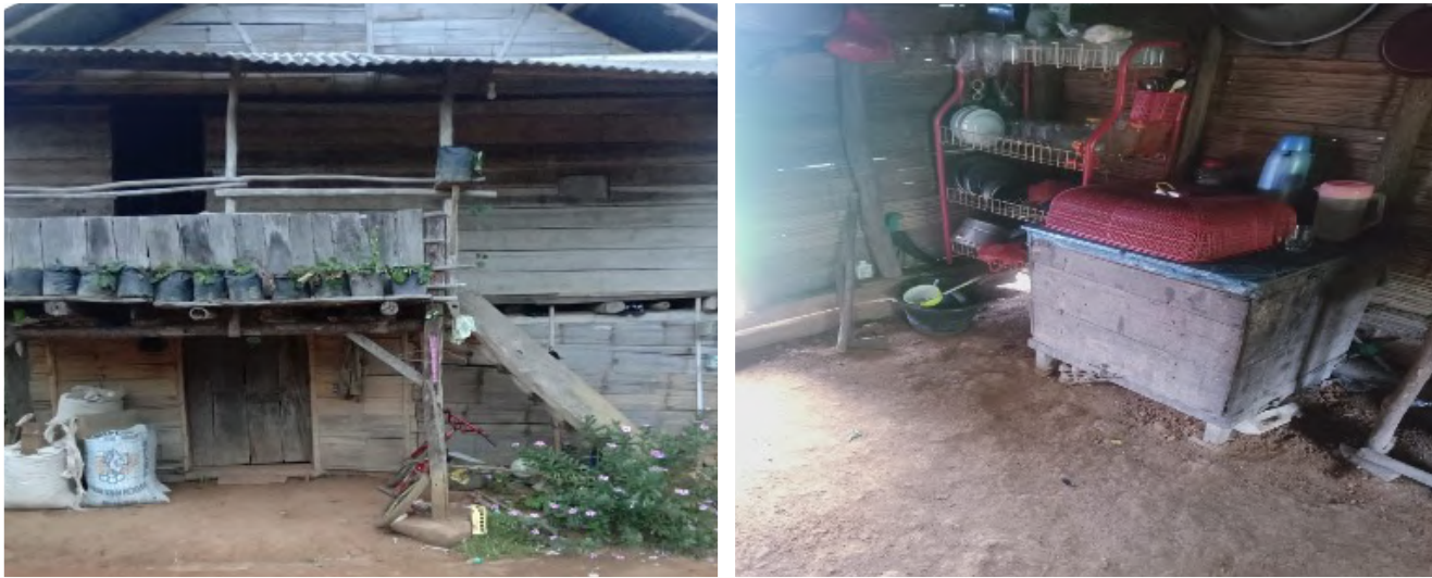
Figure 17. Unacceptable housing standard
